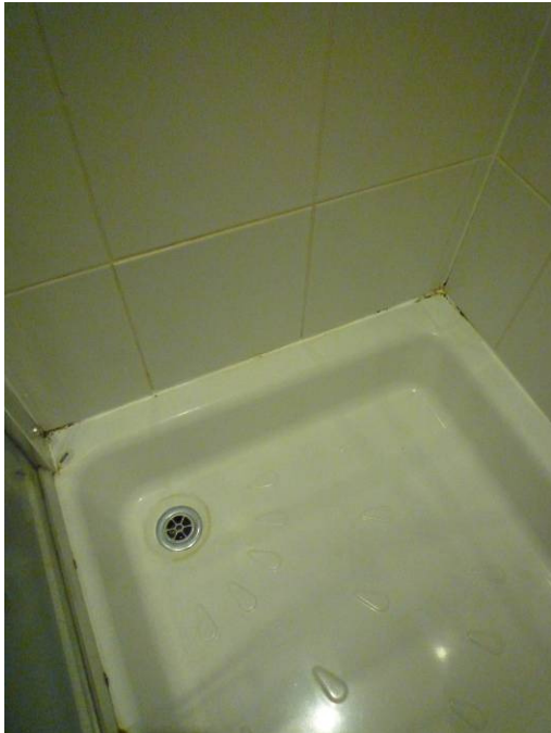
Limescale and soap scum between grout
